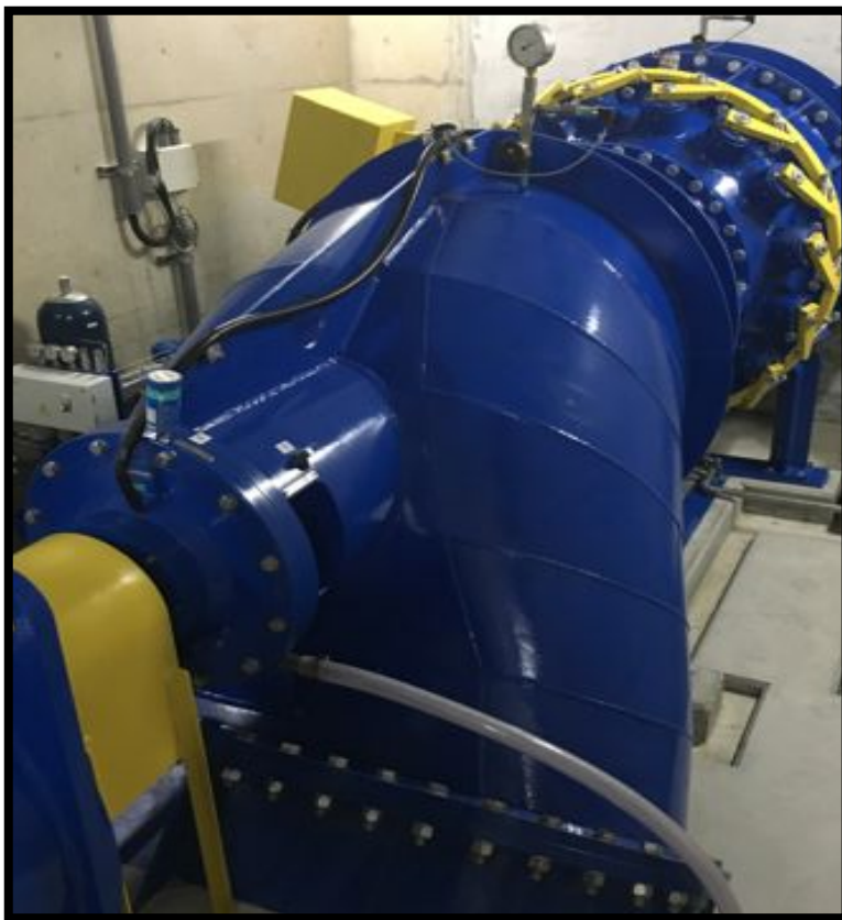
Mavel Kaplan S Model KS850K4 installed in the Yamada HPP Powerhouse
