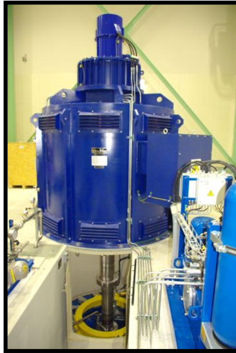
Mavel Turbine installed at the Shin Hayatsuki HPP
