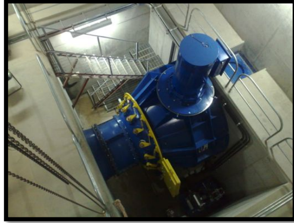
Mavel Kaplan Bulb Turbine installed at the Nakano HPP Powerhouse
